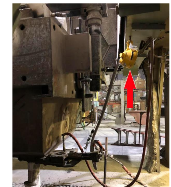
Added a winch to pull the chop block into place. Reducing the need to manually put the block into place.
